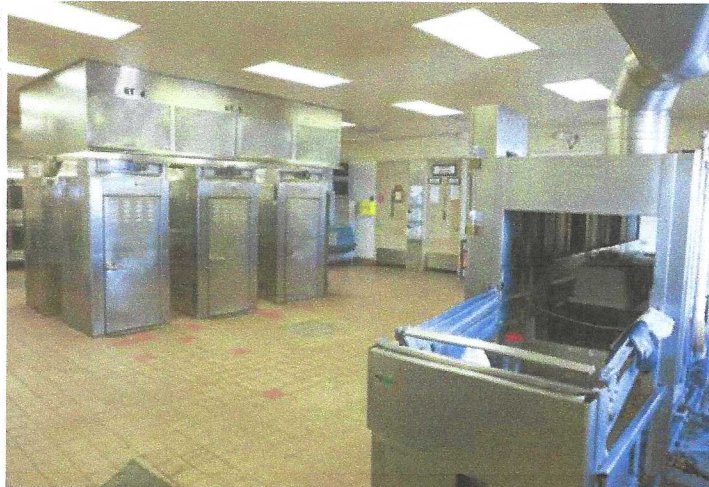
The kitchen at Avenal State Prison in Avenal, Calif., has been operating under stricter measures for all staff and inmate workers issued by the CDCR.
